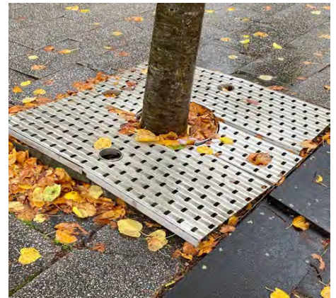
Existing trees along Newtown Square showing signs of tree root egress which is lifting the paving within the canopy diameter of the tree. Some areas of paving have become a trip hazard as a result.
