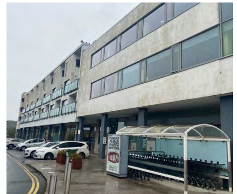
Development at Newtown Square is showing signs of wear, along with the block paved carriageway which is failing at key junctions due to stress by vehicles.
