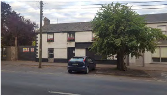
Photo (above): Example of poor building condition on the Main Street.
