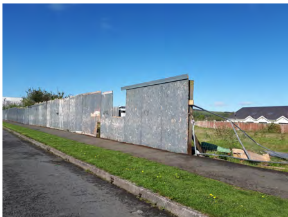
Photo (above): Site/construction hoarding which has rotten and has collapsed and requires follow up with landowner due to health and safety concerns and poor general appearance (UD6).
