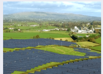
Dale Farm, example of Community Solar Farm
